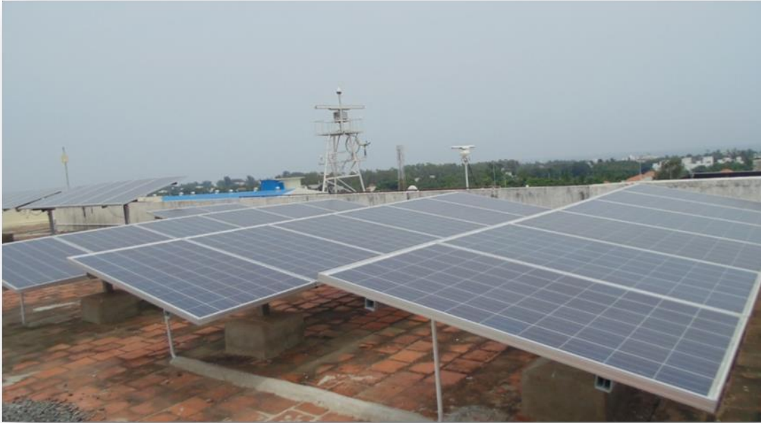
SOLAR POWER PLANT 30 KVA – RABINDRA NATH TAGORE BLOCK
